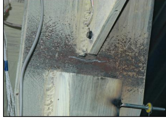
(e) Crack in knife plate(LC-2tp)[4]
